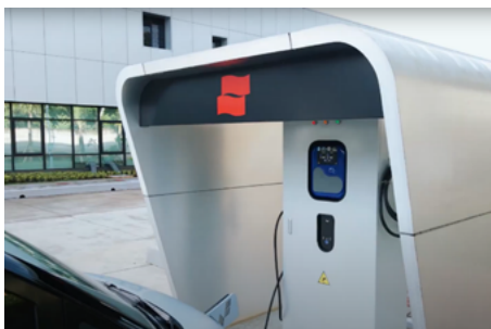
Electric vehicle charging station
